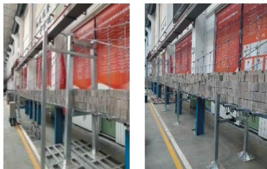
(a) 中塔塔顶测点 (a) Middle tower-top measuring point (b) 全跨加劲梁测点 (b) Full-span stiffening girder measurement point
